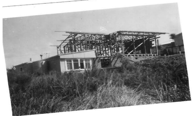
Construction began on the house, the bach retained below on the left. (Baches are considered an iconic part of N.Z.'s history.)
